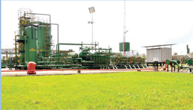
Amukpe Flow Station
